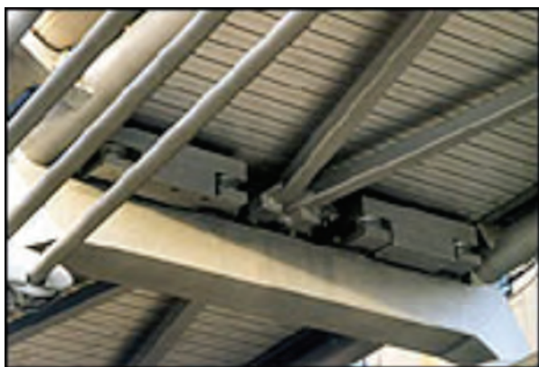
Fig. 13: Tuned Mass Damper la Millenium Bridge [w2]
